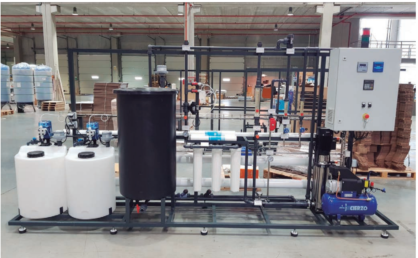
Industrial Reverse Osmosis of 43.000 l/day for the purification of drinking water in a chicken farm installed in Lérida (Spain).
