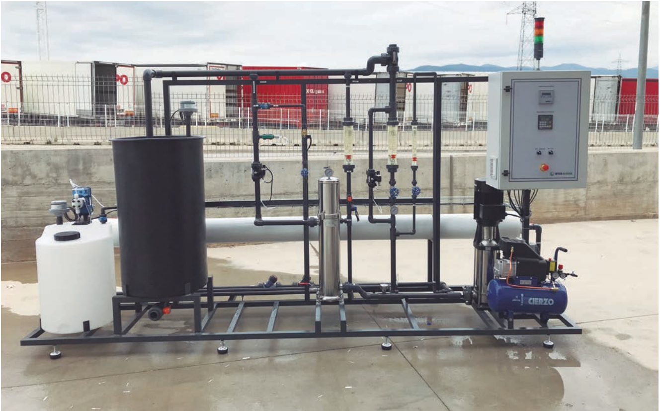
Industrial Reverse Osmosis of 60.000 l/day installed in Argelia.
